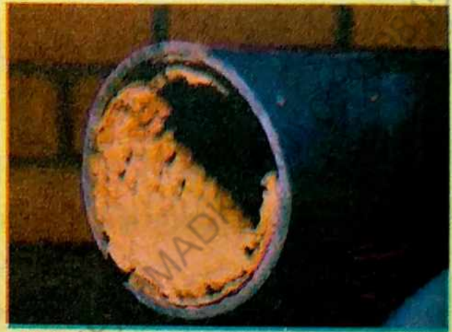
Fig. 15.5: Salts deposition inside of boiler pipes
