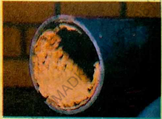
Fig. 15.5: Salts deposition inside of boiler pipes
