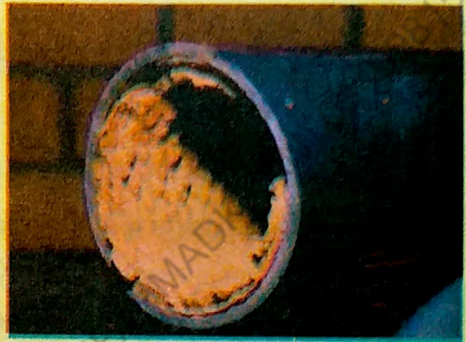
Fig. 15.5: Salts deposition inside of boiler pipes
