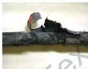
Fig: 15.23 Over heating of a cable
