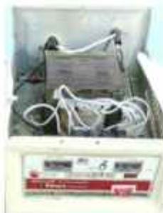
Fig: 16.20 Transformer in stabilizer
