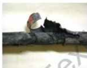
Fig: 15.23 Over heating of a cable
